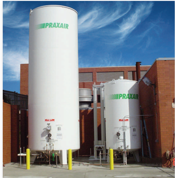
Figure 12: Medical Gas System
